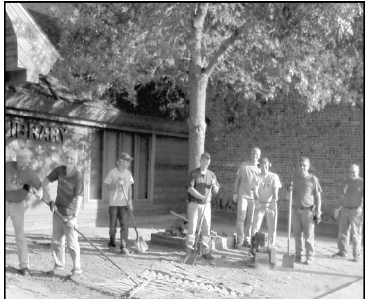
New York Mills Lions Club members worked at leveling off the surface layer of sand before replacing the original bricks outside the city's library.
